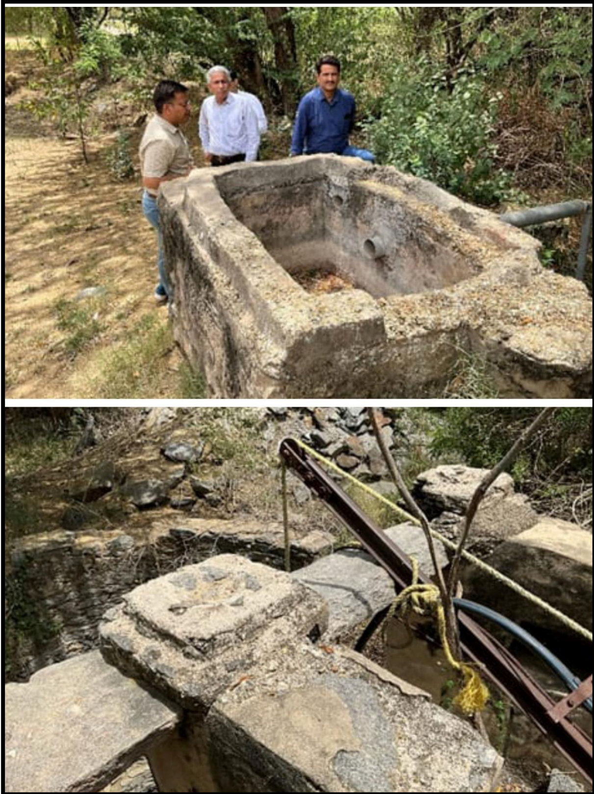
Fig 3.6: Wells present in RIE campus
